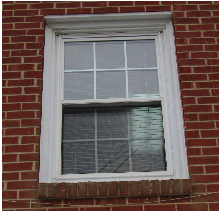
Photo 23: Replacement Vinyl Window on St. Paul's Church Addition.
